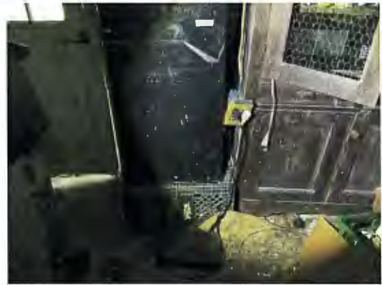
Open electrical wiring in kitchen 7/10/24
