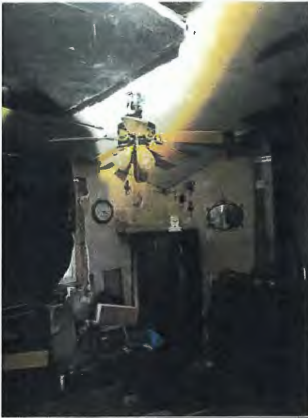
7/10/24 Failing roof TS
