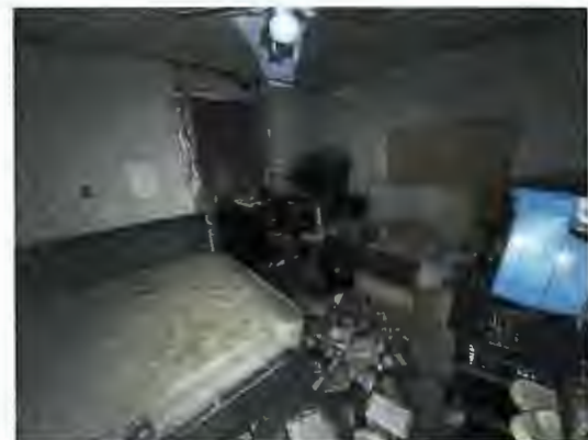
Bedroom where the hold in wall is located. 7/10/24
